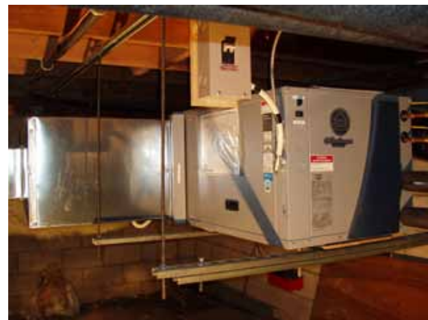
A close up of the heat pump in the basement
